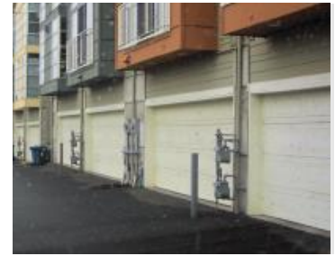
Exposed utility meters like this will not be allowed where visible from common open spaces, streets or pedestrian areas.
